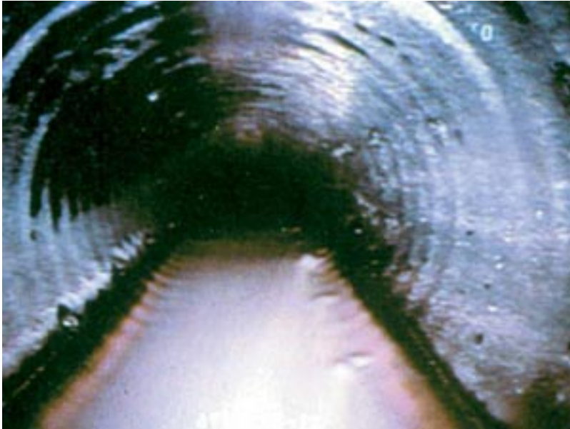
Concrete Pipe Collapse
