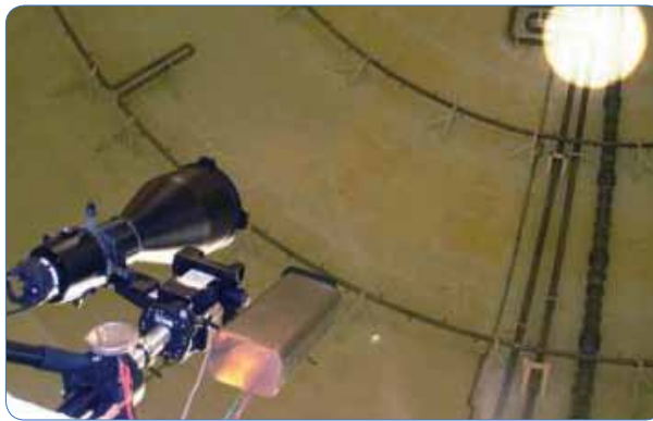
Nuclear plant containment building steel liner is visually inspected with a custom 5-megapixel imaging system to meet ASME's IWE code requirements.
