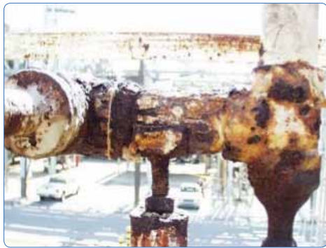
Industrial environments will promote significant corrosion of carbon steel piping components
