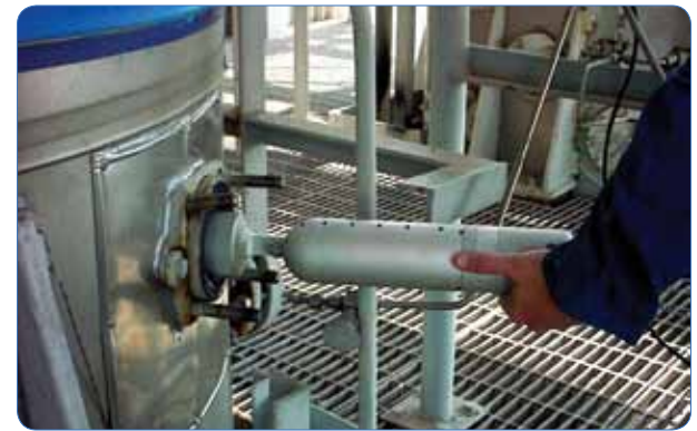
A PTZ camera system is used to inspect the integrity of glass- and refractory-lined vessels.
