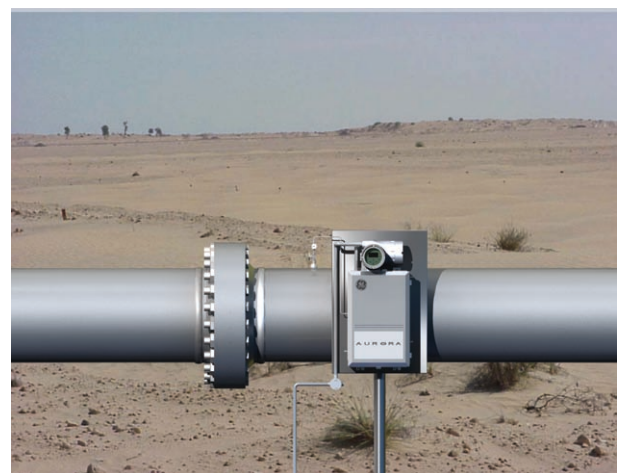
Figure 4. Aurora analyser installed on a pipeline.
