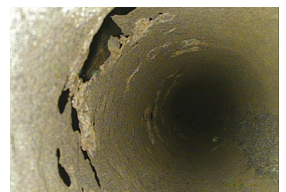
Feed Water Heater
